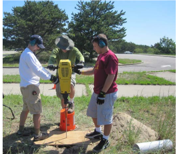
Fig. 2. Using a gas powered jackhammer to drive the steel rods into the ground (from a URI guide for installing elevation monuments on National Park Lands).
